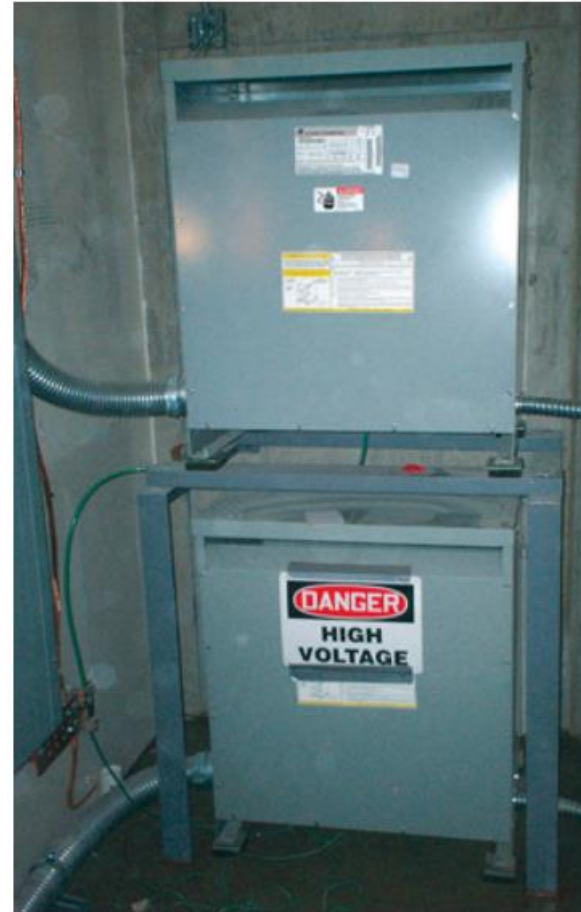
Photo 2. Two 45kVA open wound dry-type transformers in a stacked configuration.
