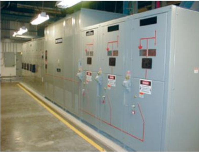
Photo 1. This 12,470V to 480V, 3-phase vacuum pressure encapsulated (VPE) transformer serving a large data center is dual rated at 2,000kVA and fan assisted to 2,666kVA. The right-hand side of the enclosure contains the medium-voltage switches, the middle section is the transformer, and the far left section contains the secondary 480V breakers.
